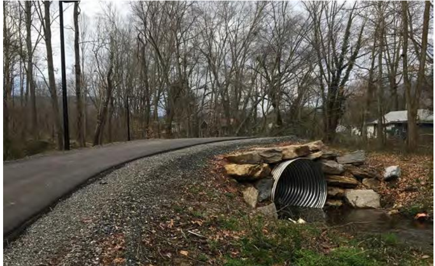
New sections of the expanding Richland Creek Greenway are designed for both functional transportation and recreation uses. They highlight the scenic appeal of the creek and its tributaries, while connecting to parks, neighborhoods, and the town's sidewalk system.
